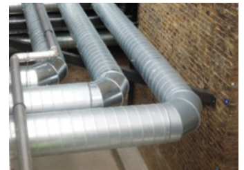
Ductwork, Ventilation and Heat Recovery
